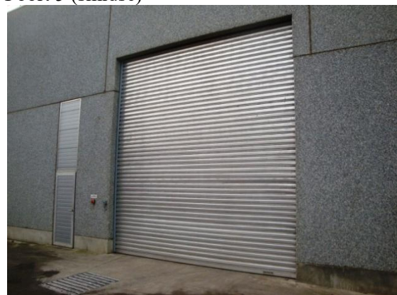
Poort stooklokaal (wateronderharder/RO)
